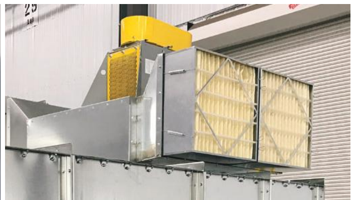
REDUNDANT FILTERS MERV 14 rated
